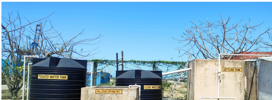
20 KLD STP at M/s. Ennore Bulk Terminal Private Limited
