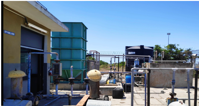
25 KLD STP at M/s. Adani Ennore Container Terminal Private Limited
