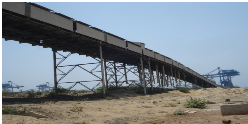
Closed elevated conveyor system
